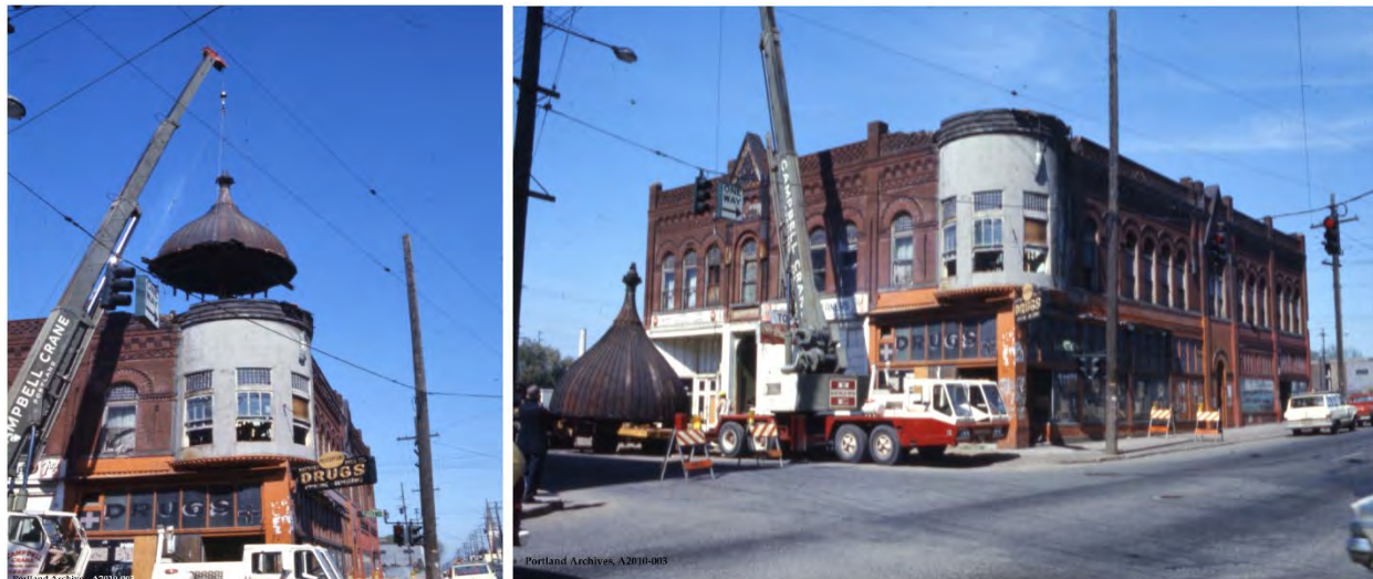
Figure 9: Demolition of the Hill Block, a building constructed at N. Williams and N. Russell by Albina's first mayor and which served as the center of Albina's business district until its destruction to make way for the Emanuel expansion project. The Hill Block's cupola was relocated to present-day Dawson Park (1973).
